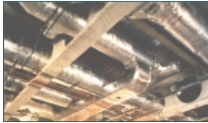
Long-span cellular beams showing full service integration and cross-over of service ducts (photograph courtesy of Westok)
