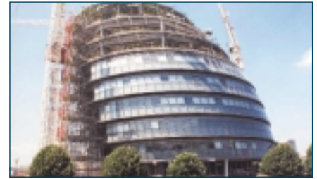
New GLA building built to high environmental specifications using traditional composite construction
