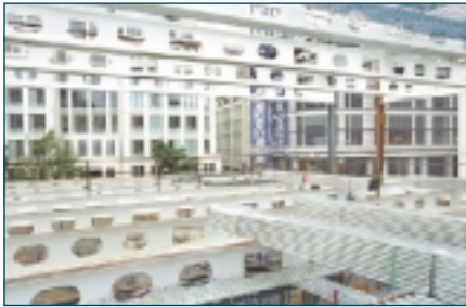
Long-span beams delivered to site with an intumescent coating (photo courtesy of Fabsec)
